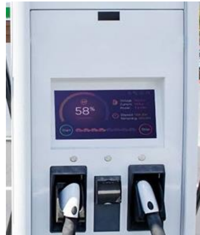
Fig. 8. EV charging performance at LCD
